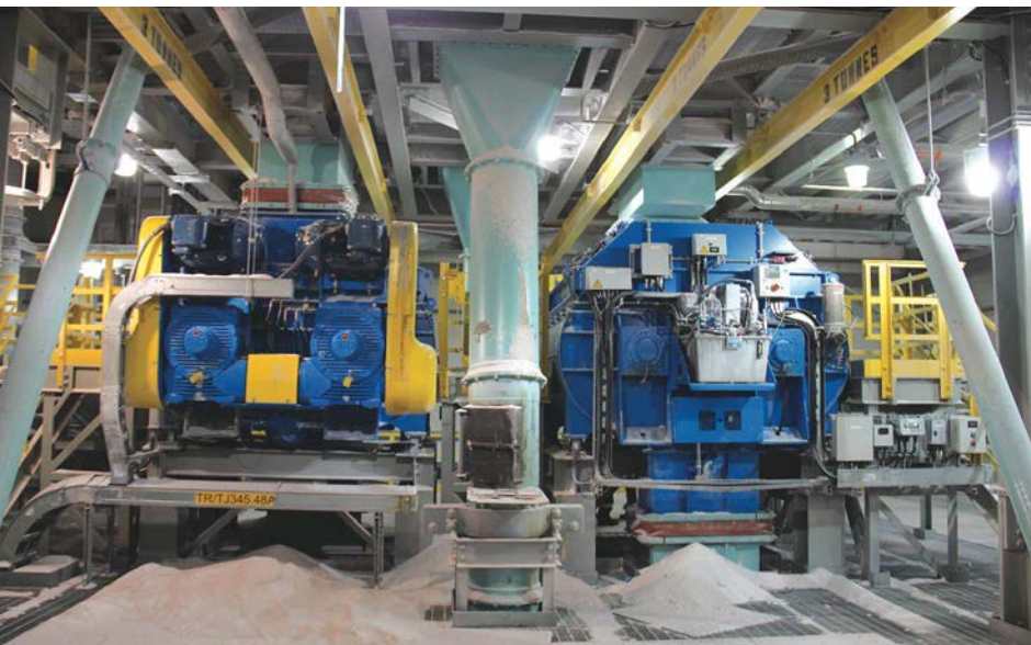
Above, two BHS-Combimix mixers, each with 65-kW drive power, process potash crude salt at the K+S Potash Canada Bethune mine. (Photo: FLSmidth)
